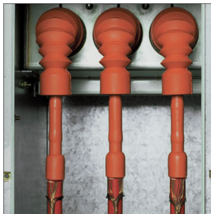
TFTI installed with Raychem bushing boot (RCAB)
